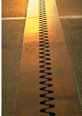
FIGURE 20-4 Expansion joints, such as this one, allow bridges to expand with increases in temperature. (Frank Siteman/Stock Boston, Inc./PictureQuest.)
