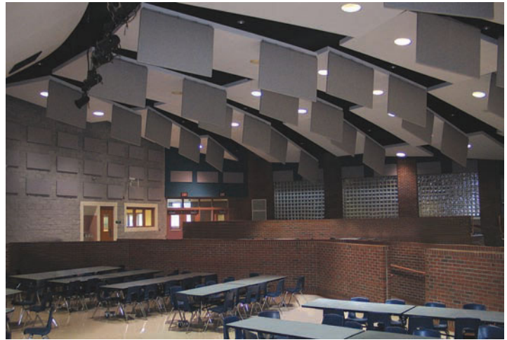
The baffles hanging from the ceiling and attached to the walls above the doorways are there to absorb sound. Their surfaces are made of acoustically dead material, like felt. (Courtesy of Perdue Acoustics.)
